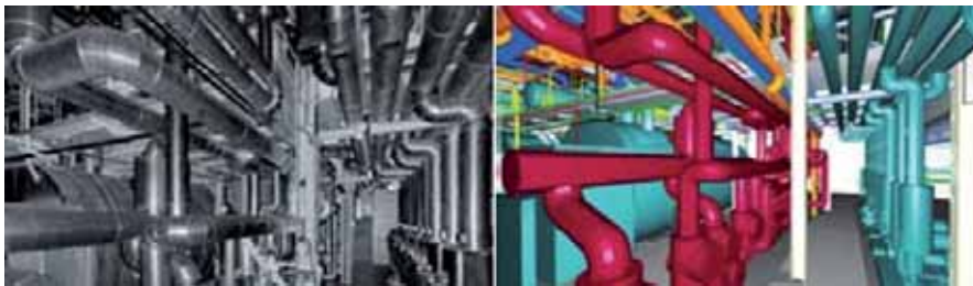
Left: Point cloud scan data. Right: the CAD model produced from the scan data
